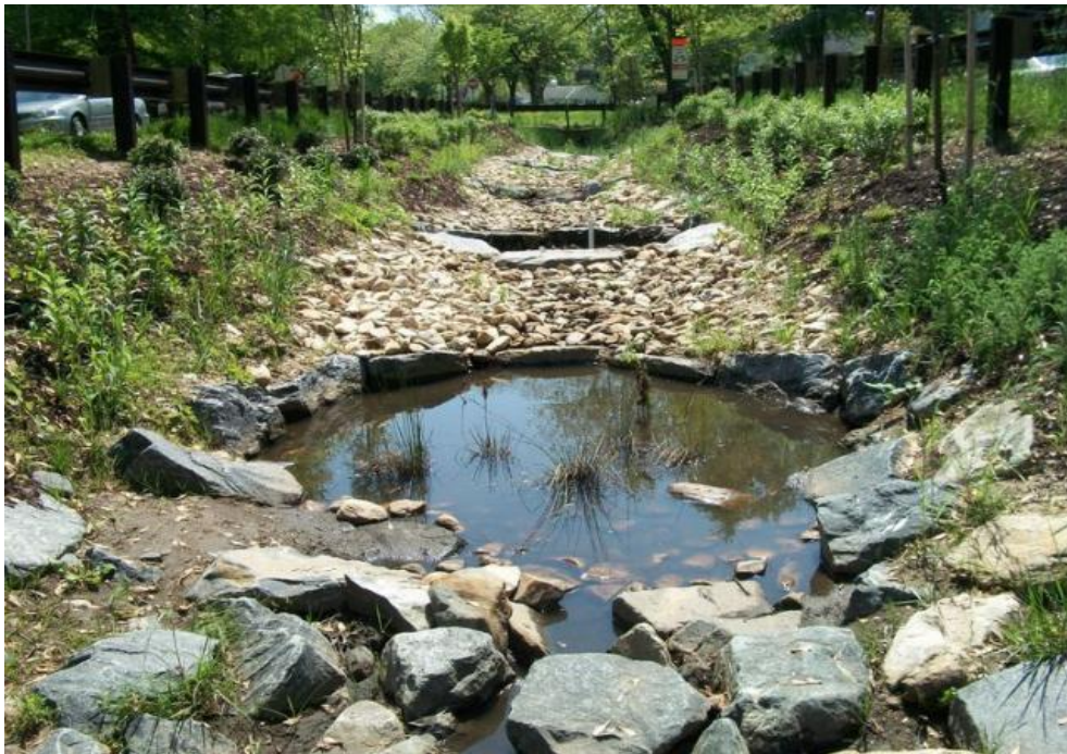
Figure 6. 10 Brushwood Check Dam
